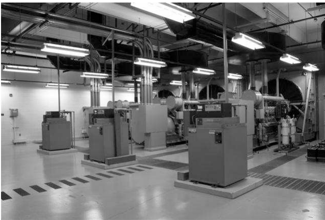
Figure 6: Microsoft Blue Ridge Generator Room
